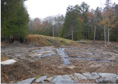
Photo 3 - #4 Green Drainage System
